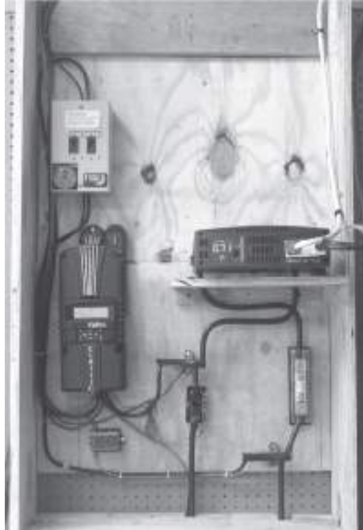
A friend's basic setup containing a solar breaker panel, charge controller, busbars, battery fuse, Whiz Bang Jr., and inverter
