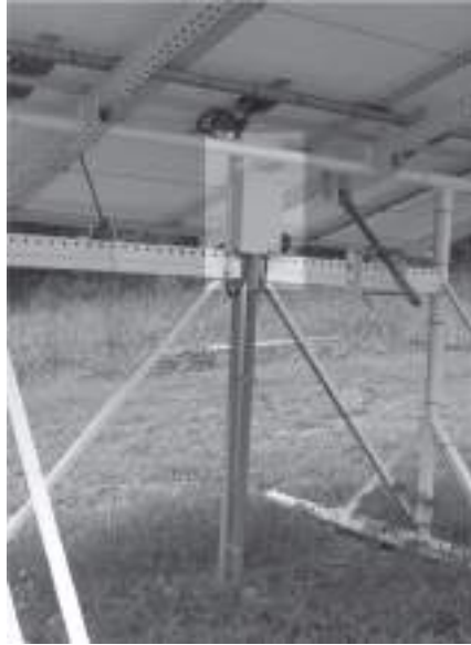
Highlighted area shows combiner box location
